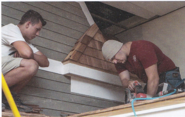
Yelsidy Bejan (right) trims a wood shingle for the roof of the house, helped by Mario Levy Adam.
